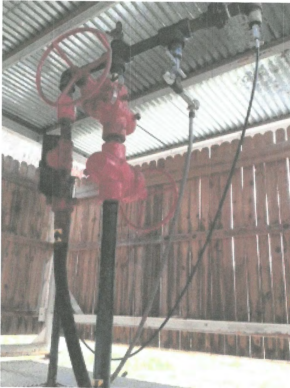
Figure 6 – BW#4 Injection Tubing with Gate Valve and Pressure Monitoring System Inside Enclosure.
