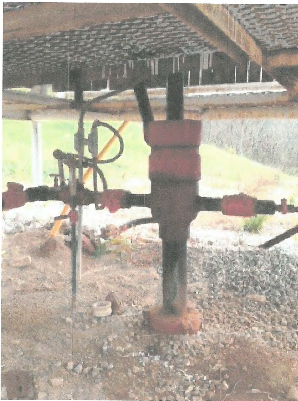
Figure 5 – BW#4 Wellhead Assembly and Annular Pressure Monitoring Equipment Below Enclosure.
