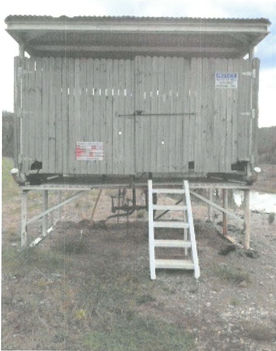
Figure 4 – BW#4 Secure Well House.
