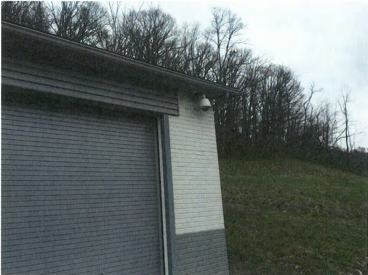
Figure 2 - Close-up photograph of 24-hour surveillance security camera.
