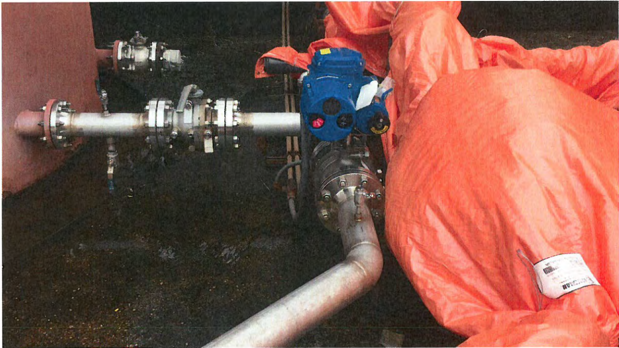
Figure 4 - Pipeline and locking valves as additional security measures.
